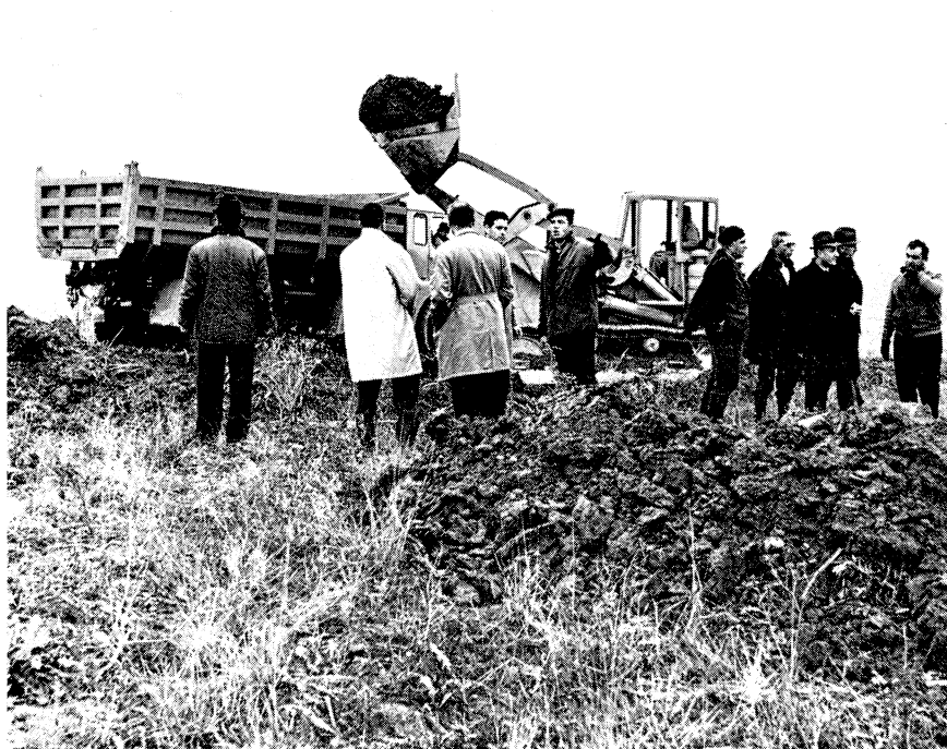
Starting on the ISR tunnel. This photograph was taken on 2 November when work began at the position of the intersecting rings on the French half of the CERN site. The earth excavated in carving out this tunnel, 15 m wide about 7 m high and with an average diameter of 300 m, will be transported to a dump on the opposite side of the Geneva - St-Genis road using a tunnel cut under the road. The earth required later as shielding around the storage rings will be stocked on the site.
